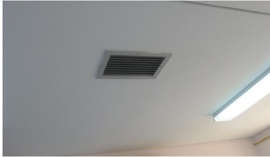
Figure 100: gypsum board ceiling: Clinical Lab, Beira Central Hospital
