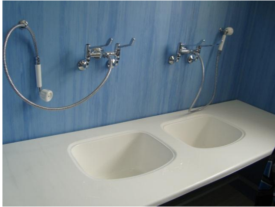
Figure 102: Wall mounted fixtures, Clinical Lab, Beira Central Hosp.
