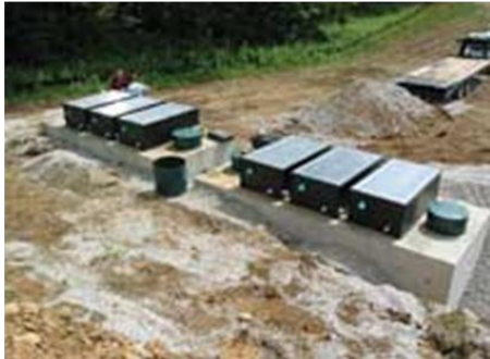
160: Onsite sewage treatment facility, Huntingburg IN
