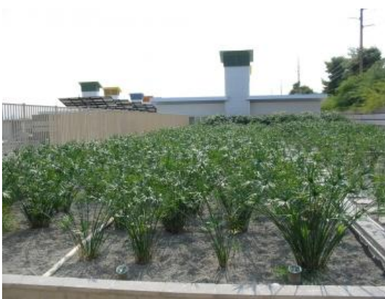
157: Wastewater treatment by a tidal flow wetland living machine system, RAC Las Vegas
